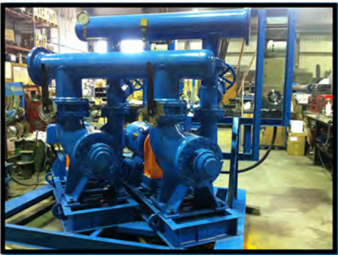
Cooling Pumps Toronto, Canada
